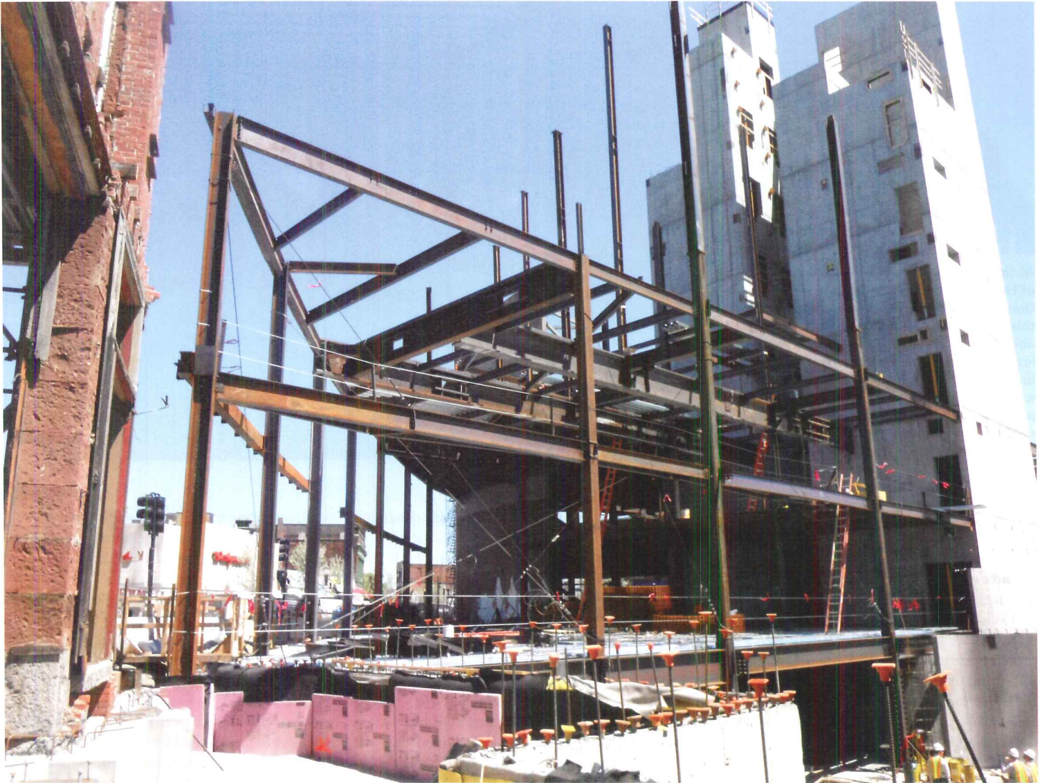
Incorporating Boston's historic Curtis and Waterman buildings, and uniting their facades with five additional stories of structural steel, Arup worked with Sasaki Associates to design this new 215,000-square-foot headquarters for the Boston Public School system.
