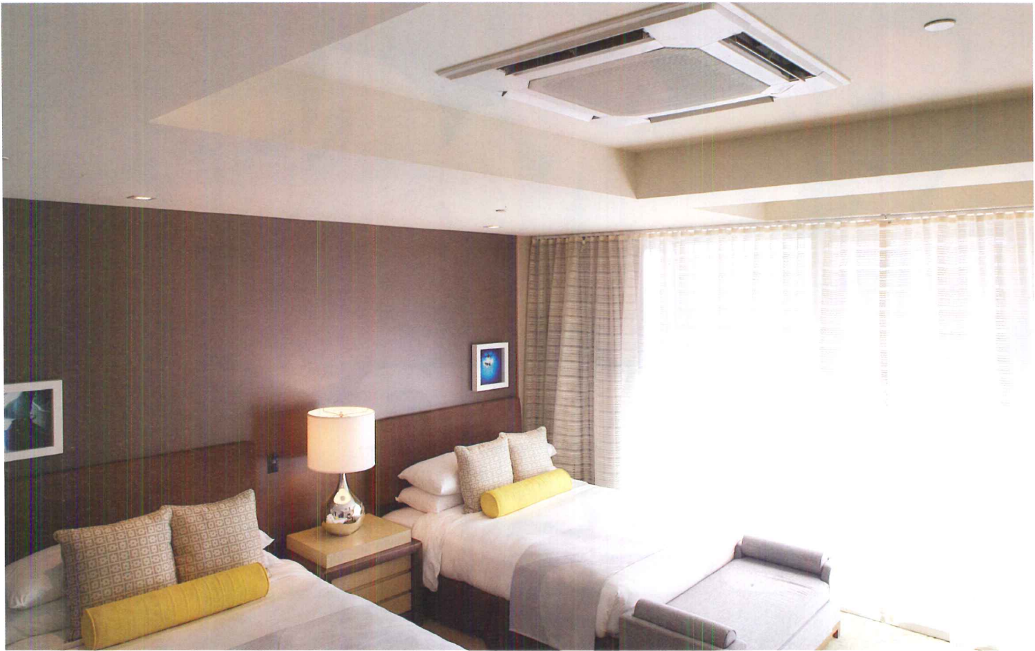
The highly energy-efficient variable refrigerant flow (VRF) zoning system was used in Hotel Wilshire, which earned key LEED credits.
