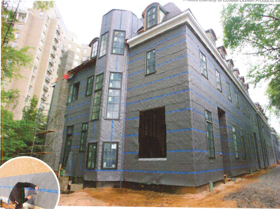
A ventilated rainscreen over a polymeric, water-resistive barrier protects the enclosure for Bellingrath Town Residences in Atlanta's Buckhead.
