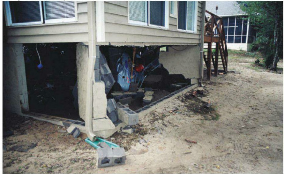
Hydrostatic pressures are extremely strong under flood conditions, and can shift, separate and even destroy foundations if not properly floodproofed.
