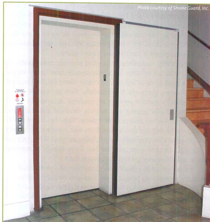
A swing door mounted at an elevator opening and held open with a magnetic hold meets the fire and smoke partition code requirements, but can be susceptible to tenant tampering and have an undesirable aesthetic effect in the space.
