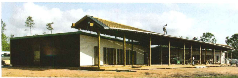
A crew completes work on two SHoP-designed buildings unified by a sculptural canopy.
