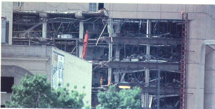
Structural damage and broken glass were major contributors to death and injury for both the targeted buildings and the surrounding area in the 1995 bombing of the Murrah Federal Building in Oklahoma City.
