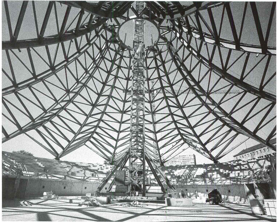
The Tempodrom in Berlin is a folded-steel-plate structure with 5-inch-thick concrete infill panels. A temporary tower was erected to support the frame during construction.
