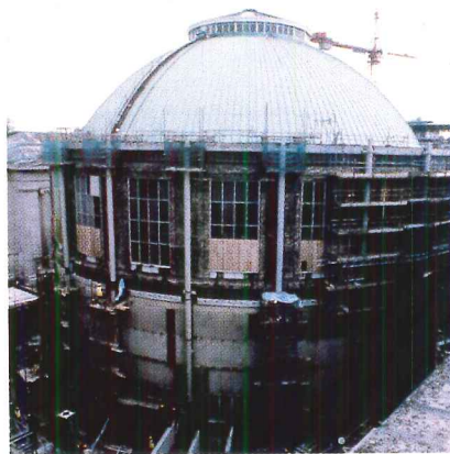
was erected. During demolition, the exterior of the Reading Room (above, right) was revealed for the
