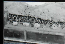
Pea gravel and straight strip products cause damming and clogging of wall cavities which result in costly repairs due to water damage.
