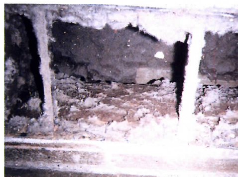
© Courtesy Ductbusters, J. May Home Inspections
