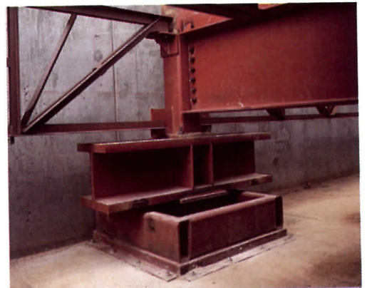
The design team chose a "base isolation" system to accommodate seismic loads. They also specified Vulcraft steel joists and joist girders for the building.
