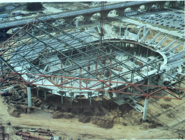
The Arena's 176,400-sq-ft space truss is supported on eight 6-ft-diam columns. The roof has a 412-ft clear span and overhangs the substructure by 4 ft on each side. The frame's corners cantilever 70 ft from the column line.
