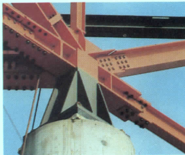
Steel box sections embedded in 5-ft-high column caps are bolted to the space truss with 3-in.-diam anchor bolts. Four-foot-square elastomeric pads accommodate rotation at each connection.
