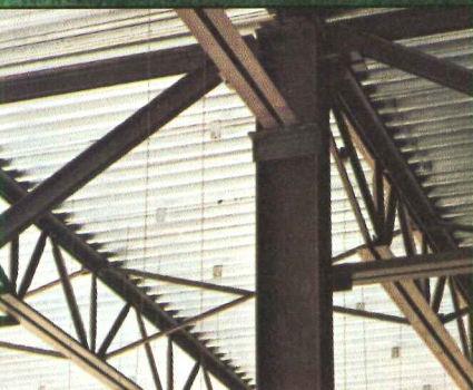
The efficiency of Vulcraft's standardized column speeds up steel erections and saves costs.
