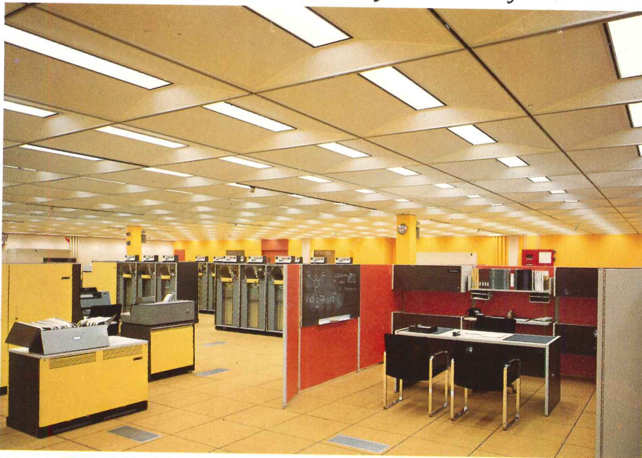
Datacenter/The Equitable Life Assurance Society of the United States, Easton, Pennsylvania, Architects: Kahn and Jacobs, New York City, Ceiling System: Armstrong C-60/60 Luminaire
