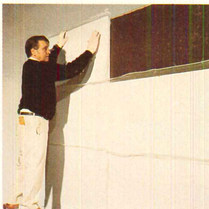
A plasterer demonstrates the ease and simplicity of the Thermoclad system, applied here over an 8 x 8 foot panel of exterior gypsum over metal studding. In the first photo, Thermoclad insulation
