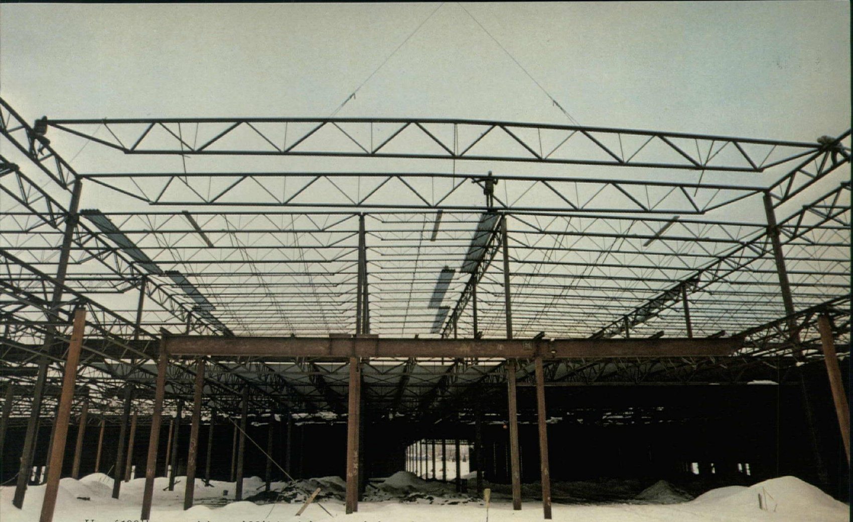
Use of 100' long span joists and 30' joist girders created a large clear span area in the center section of this enclosed shopping mall.
