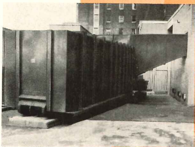
Through-the-wall loading in to a Dempster Packer provides a convenient, all-weather refuse disposal system.
