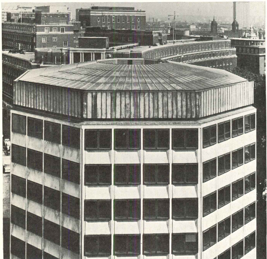
The fascia of the roof of this six-story building is in the form of an open screen comprised of 200 panels of lead clad steel. The panels are fabricated from 20 gage steel with a lead coating of about 1½ pounds per sq. ft. (.0234" thick) on each side.
