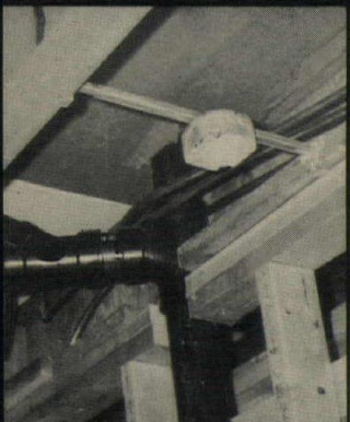
Accommodate even large duct work.
