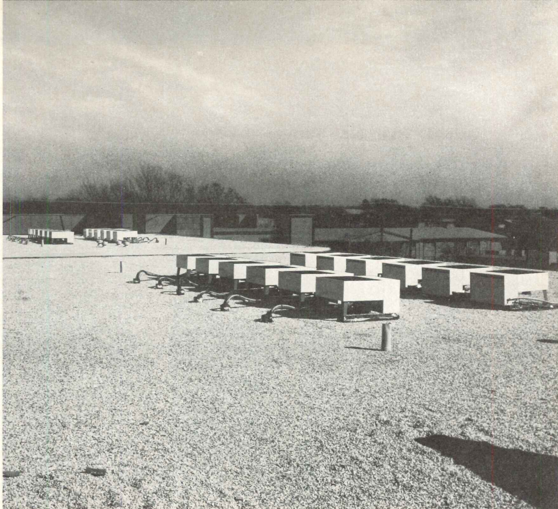
Mi Amigo Apartments, under construction in Dallas, is a complex of 149 apartments with individual ducted Lennox heating and air conditioning. New-design cooling units hide low on the rooftops. Architect: John Moss. Building Contractor: GTC Company. Heating/cooling contractor: Citywide Plumbing & Air Conditioning. Owners: George T. Connell and M. I. Harris, Jr.
