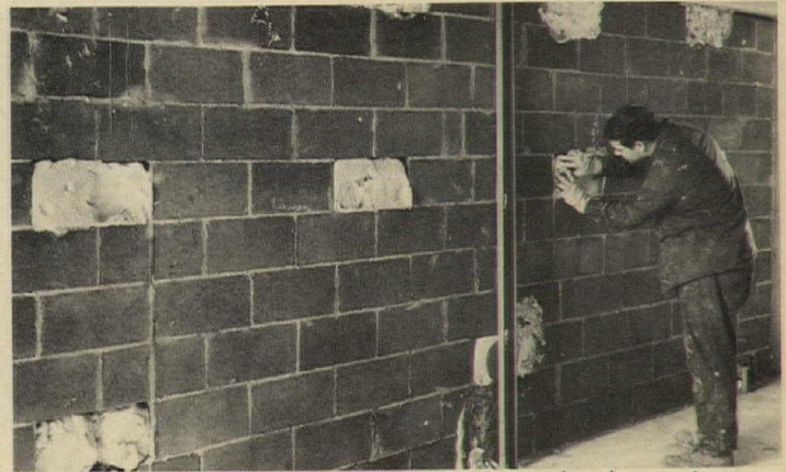
The foam expands so as to not only fill the wall cavity but the openings as well, assuring that the cavity was completely filled.
