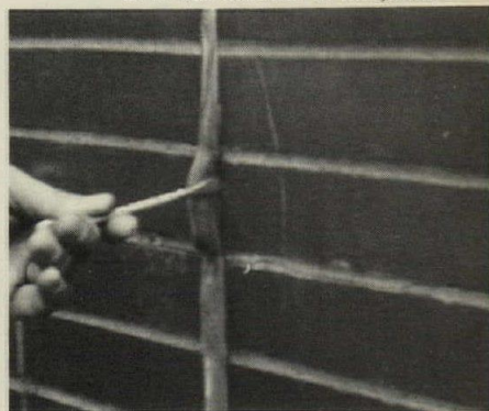
Presence of moisture behind brick wall caused "reversion" of sealant (becomes gooeey again). Joints should be vented to avoid this
