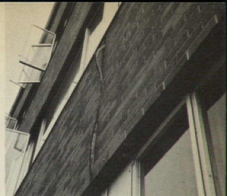
Sealant was pushed out because the back-up material had been twisted as it was inserted in the joint.
