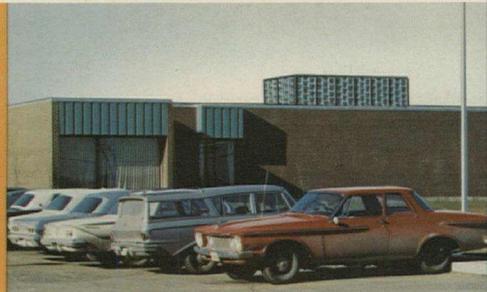
AFTER Titus Decorative Enclosures. Equipment is covered, enclosure blends into color and lines of building.
