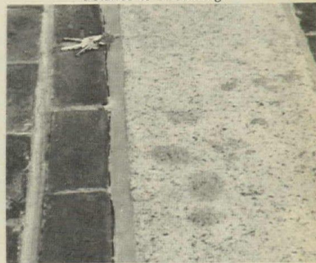
Adhesive failure of this pavement joint was caused by the high modulus (stiffness) of the sealant.
