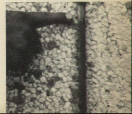
Below: Dirt "attracted" by sealant soiled aggregate near joint. (Note dirt wiped off by finger.)
