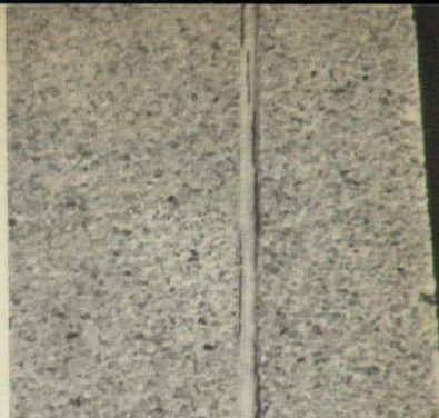
Sealant failed cohesively and adhesively. It probably had too much resistance to stretching.
