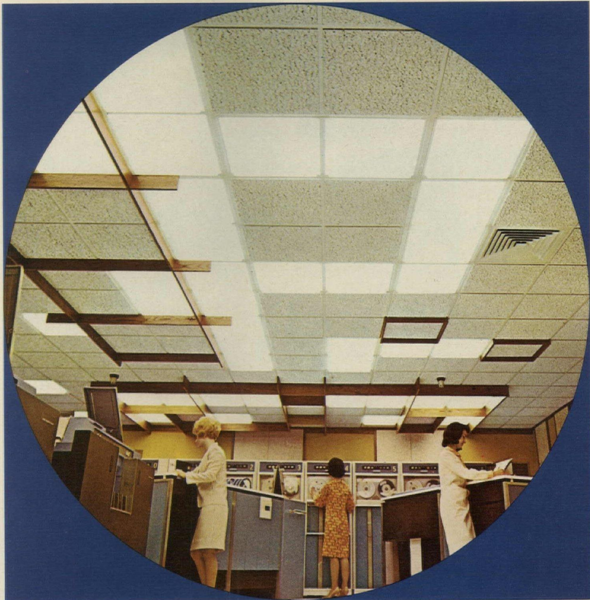
Data Processing Center, Continental Telephone Co., Wentzville, Mo./Architect: George Quick, St. Louis/Acoustical Contractor: Lindberg Acoustics, Inc., St. Louis.
