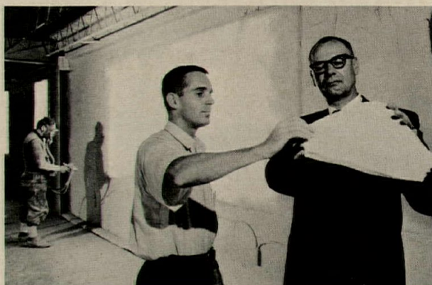
M. Tulou, who supervised installation, and owner B. Gordon examine cured urethane foam section from wall surface.
