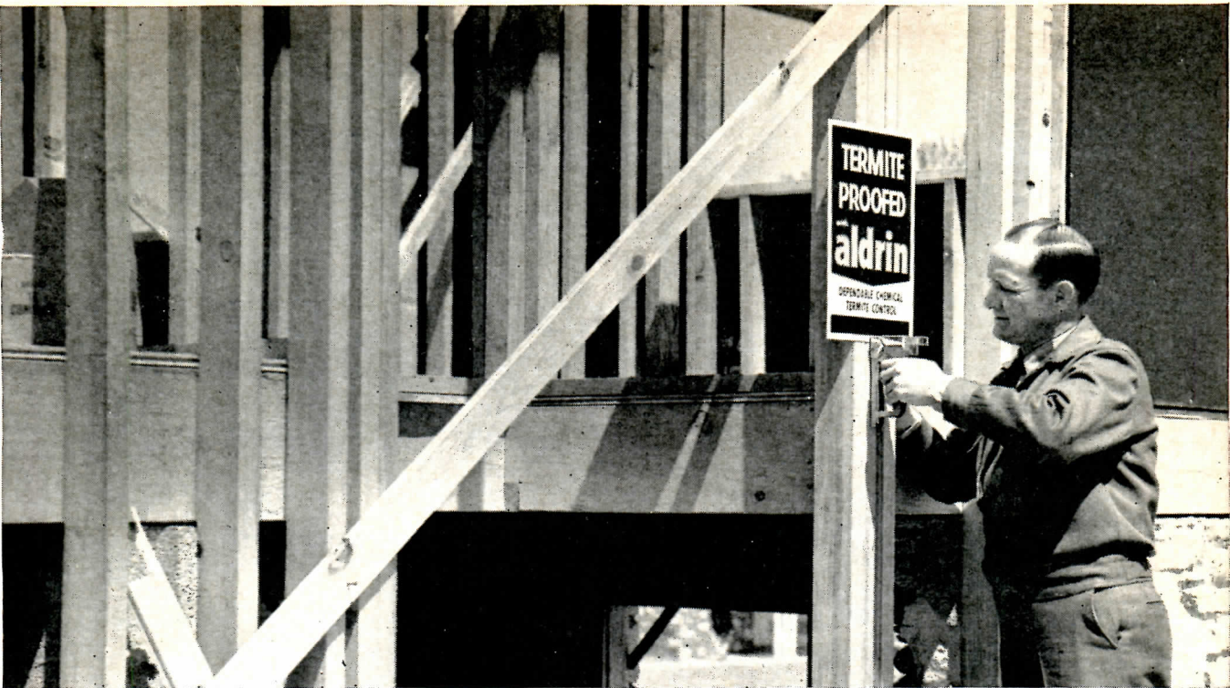
A professional pest control operator can termite-proof a building for more than 15 years with a single application of aldrin.
