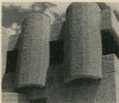
Paul Rudolph: Endo Laboratories, Long Island, N. Y. Under construction. David Attie photo
