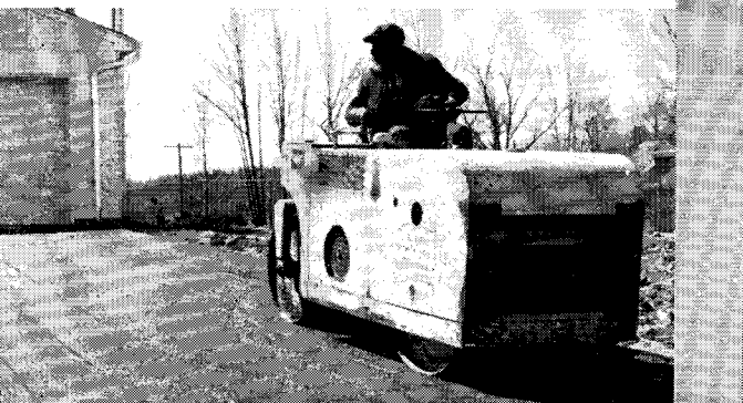
FINISH-ROLLING the black top. Note how embedded Revere Copper Water Tube readily withstands the weight of this large roller.
