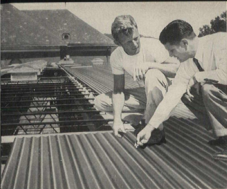
Deepest corrugation , \frac{3}{8} -inch, of all standard steel centering is available with Fab-Form. Job Superintendent Thomas A. Laboon, left, shown with Pittsburgh Steel Products Salesman C. W. Bainbridge Jr., said deep corrugation helped make a stronger slab.
