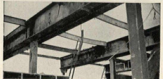
The proof of the pudding! After a fire in this warehouse, primary girders, protected by SPRAYED "LIMPET" ASBESTOS, remain in perfect condition. Unprotected purlins buckled.
