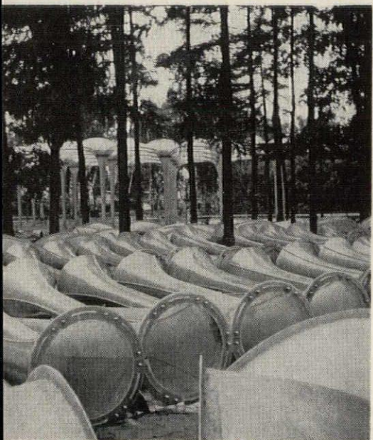
As shown above, ninety canopy sections were shipped to and assembled at storage area before being joined to columns and erected in clusters. On-site assembly, which went on while site was being prepared and footings placed, consisted of joining the six doubly-curved shells in each canopy to the steel spider and to each other. Large holes in flanges of radial ribs were field-drilled for more accurate fit. Already-erected cluster in background of lower photo is pavilion for fashion show
