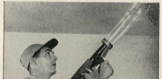
Applied in one operation! Gun sprays dry asbestos fibers which combine in mid-air with water spray.
