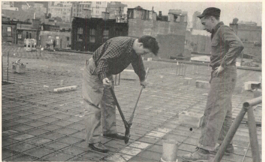
On first floor, mats were placed on top of boxes, sleeves, vents, etc. and cut away where necessary. To speed steel placement, mats on subsequent floors were laid first, as above, and cut-outs for slab breaks were later made in locations indicated by markings on forms
