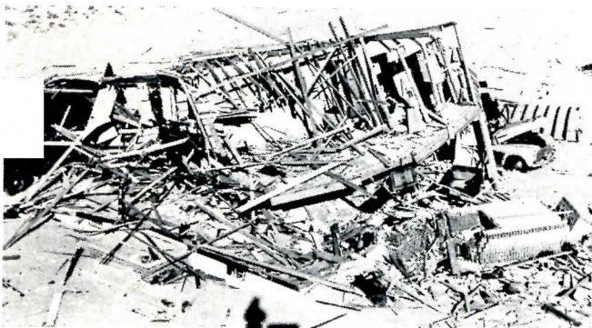
WOOD — Two-story frame house; 5 psi overpressure
