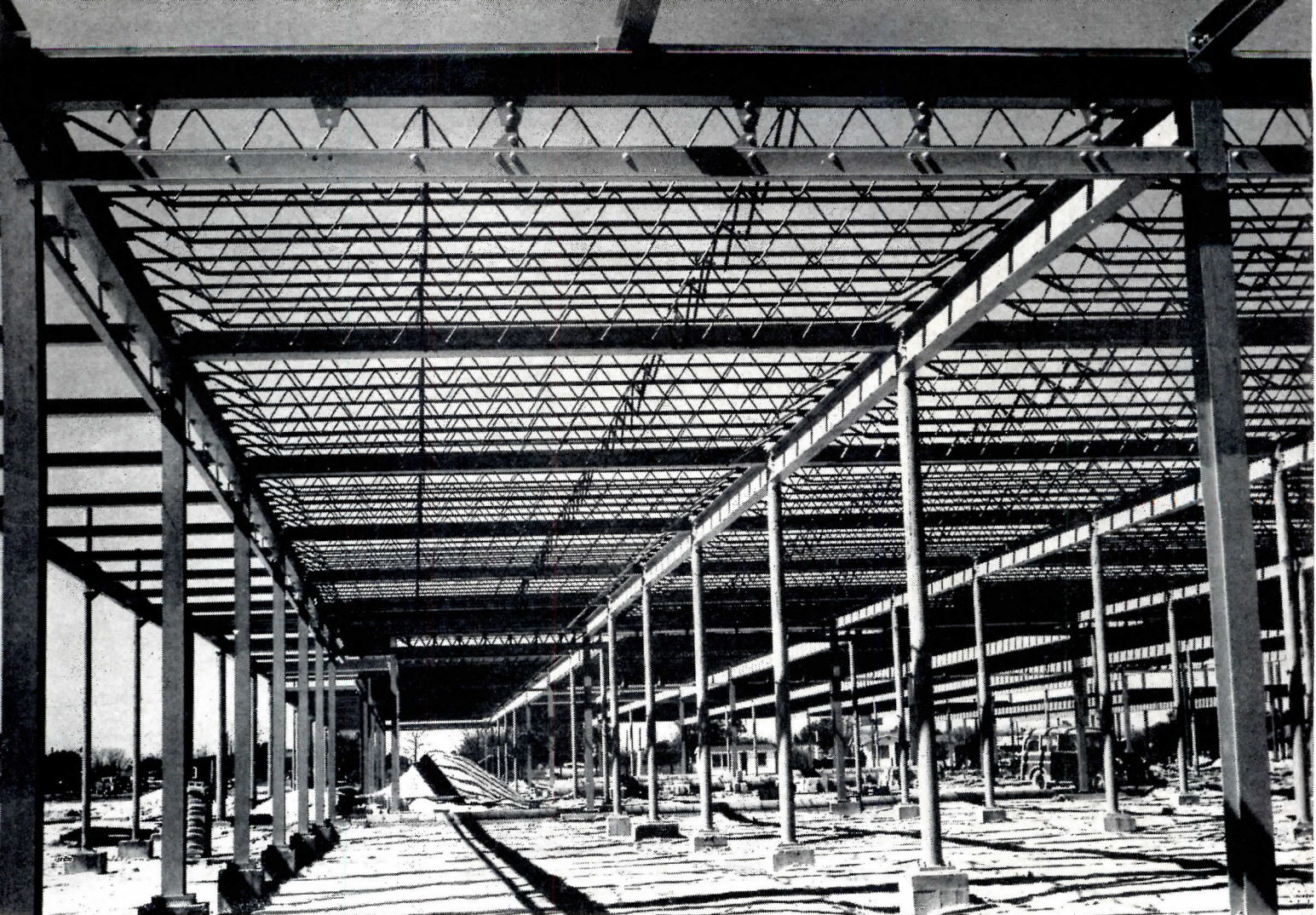
THE TOWN AND COUNTRY PLAZA SHOPPING CENTER, Pensacola, Fla., used 1,825 tons of structural steel, including 448 tons of AmBridge Steel Joists —all fabricated and erected by American Bridge.
