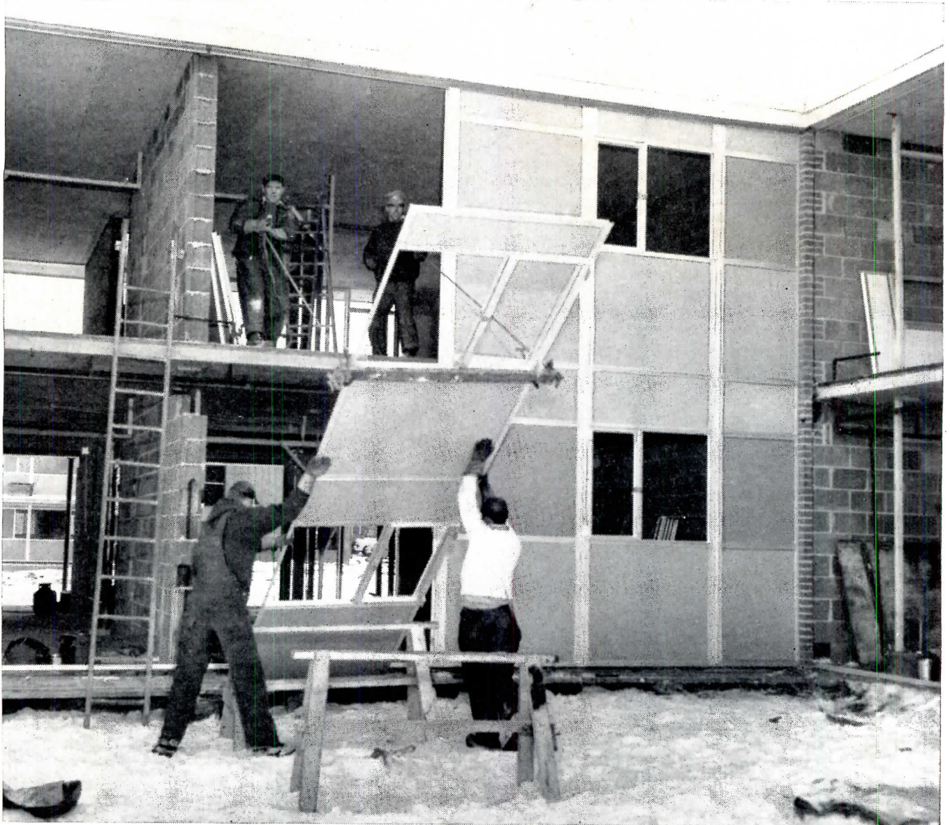
Workmen installing window walls made with Hasko-Struct † plastic laminated sandwich panels. Architect is Manson & Carver Associates, General Contractor is Christman Company.
