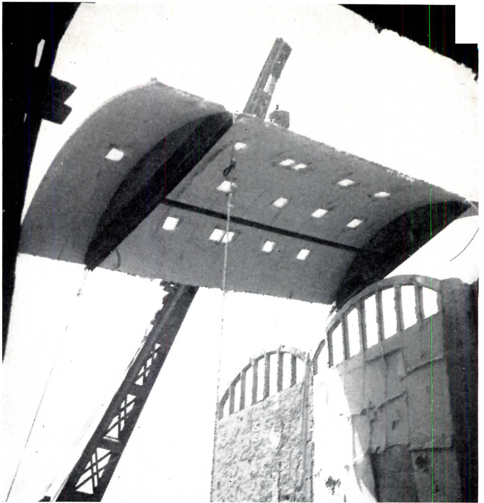
Openings for doors and windows — and even glazed skylights as in the shell at right — are formed into the elements as they are cast. To eliminate tie rods and speed erection, column capitals and upper wall sections follow the curvature of the shells they support.
