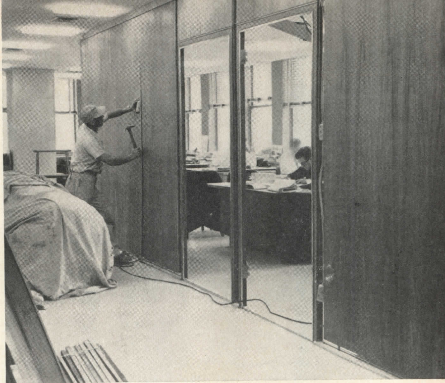
PARTITIONS ARE INSTALLED without costly interruption of regular office routine. Workman is shown installing section of Weldwood Movable Partition; completed corridor is shown at left.
