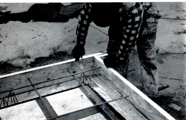
DEFORMED steel reinforcing bars (1/4" to 5/8" depending on panel area) are wired onto "chairs" to keep them about 1/2" above the bottom of the panel face.
