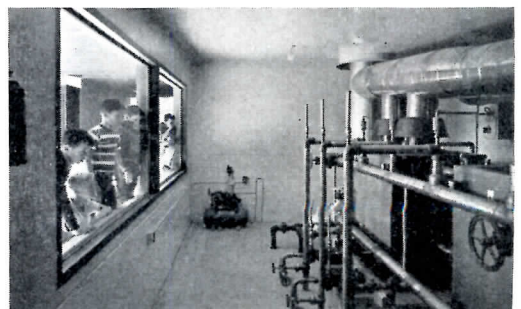
Heating plant serves educational ends
