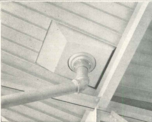
Mahon Steel Deck Roof Installed on new Lincoln-Mercury Plant, Wayne, Mich. Giffels & Vallet, Inc., L. Rossetti, Architects and Engineers. Bryant & Detwiller Co., Contractors.
