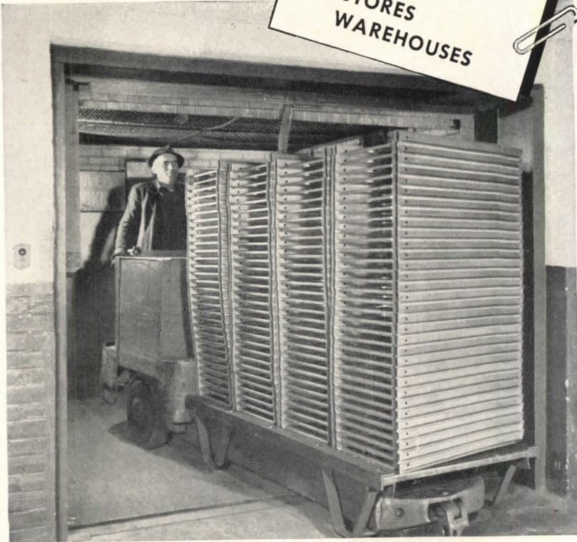
This Globe Elevator carries 15,000 lb. loads between 3 floors in a Philadelphia factory. It is a perfect illustration of the simplicity of design that makes Globe America's most economical elevator.
