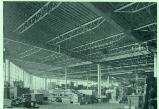
Standard joists span up to 32 feet and Long-span joists up to 64 feet. By using these maximum spans, the number of columns are reduced and more manufacturing area is made available.
