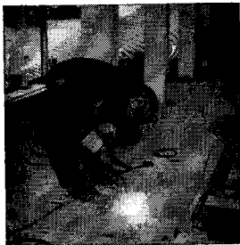
Fig. 2. Welding type D Fenestra panels with Lincoln "Fleetweld 5" electrodes. Total dead weight of floor including ceiling and finish surfacing is only 14 lbs. per square foot.
