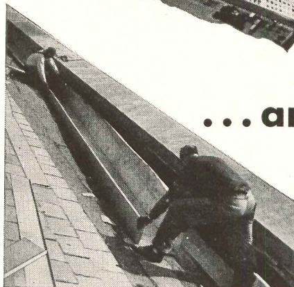
INSTALLING A RIVETED AND SOLDERED section of Monel Roofing Sheet in the built-in gutter of the Pentagon's outer perimeter. Fabricator, Rupertus Sheet Metal Works, Washington, D. C., reports: "Some of the gutters were 55 inches in girth, but Monel was easy to fabricate and install."
