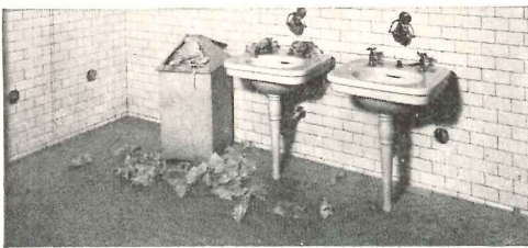
Note towel litter and disposal unit. A fire hazard.
