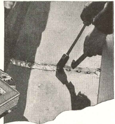
FOR PERMANENT PROTECTION, the old gutters have been replaced with gutters made of strong, corrosion-resistant and economical Monel Roofing Sheet. Here a worker solders a riveted seam in the gutter lining.
