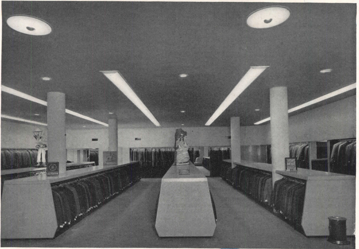
Men's Clothing Dept., Greenfield's Store, St. Louis, Mo. Five continuous rows of nine fixtures each are recessed in the 11'2" ceiling to produce approximately 40 foot candles maintained. L-I-N-O-L-I-T-E Series 17 two lamp troffers with curved Holophane Controls (17-248) were used for this installation. Architect: Meyer Loomstein.
