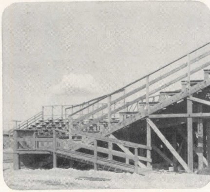
2. Ground moisture and rain held in joints, etc., of outdoor structures.
