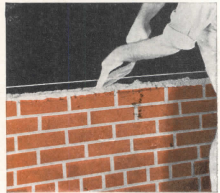
Mortar for this bed joint was spread out on the wall too far.
