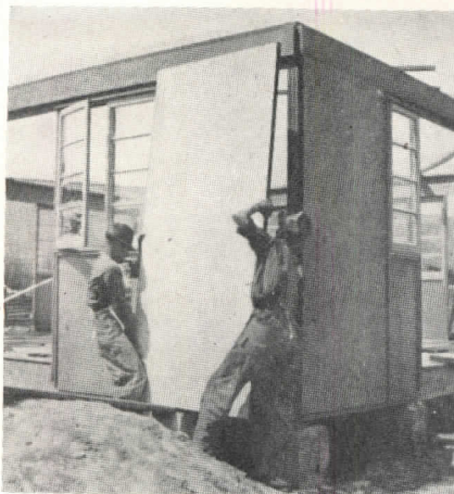
Insertion of insulated wall panels in a prefab. From "The Prefabricated House"
