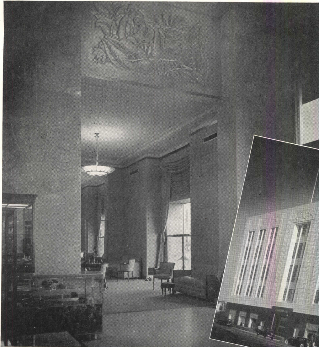
(Left) Typical richly decorated display room. Note conditioned air supply grille below frieze. Western Air & Refrigeration, Inc., designed and installed the system.
