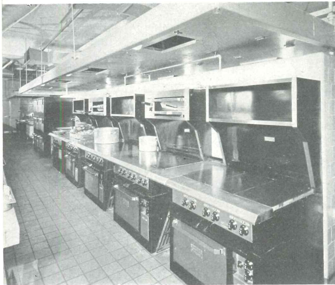
Carefully vented battery of ranges in the view below is to be seen again in the background of the view above. The size of the plant kitchen depends on the size of the total work force and not, like the dining rooms, on the largest shift
