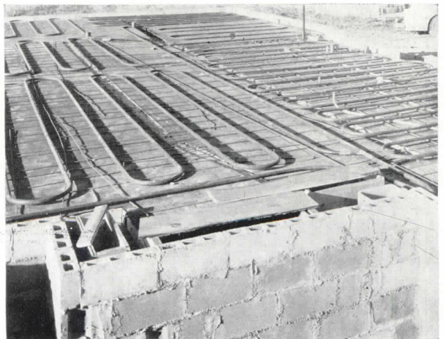
Pipe coils anchored in place above the reinforcing bars and ready for the fill and concrete to be poured
