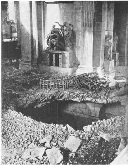
St. Paul's Cathedral has been hit twice by high explosive bombs. This view shows the north transept, where the debris caused the church floor to collapse into the crypt. Neither direct hit has interfered with the stability of the structure as a whole. Photograph from "The Bombed Buildings of Britain"
