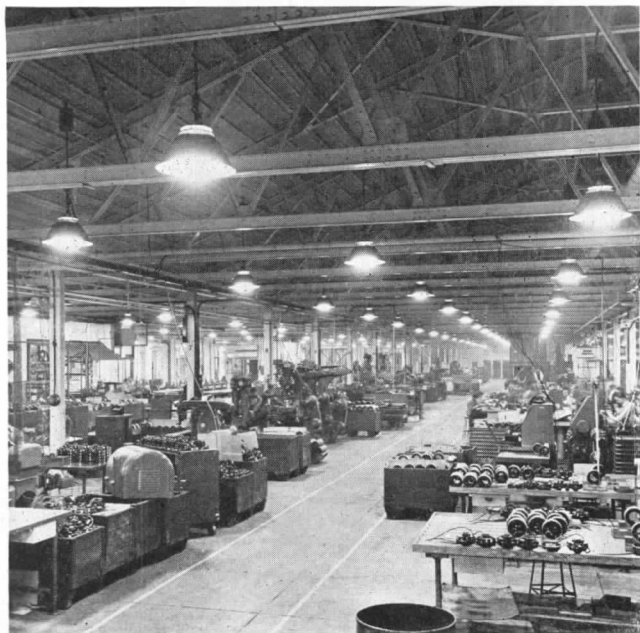
Combination mercury installation. Each unit uses one 250-watt high-intensity mercury lamp and three 100-watt incandescent lamps. It provides 20 foot-candles upon working surfaces
