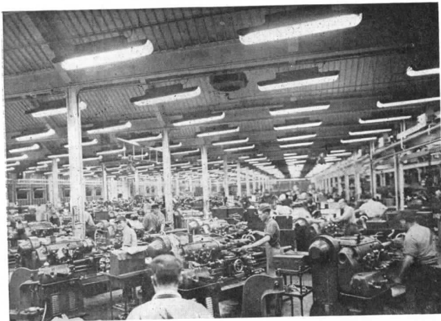
The maximum utilization of floor space is accomplished by well distributed lighting. The system employs 2-lamp fluorescent units on 10 ft. by 10 ft. spacing, 12 ft. and 13 ft. high
