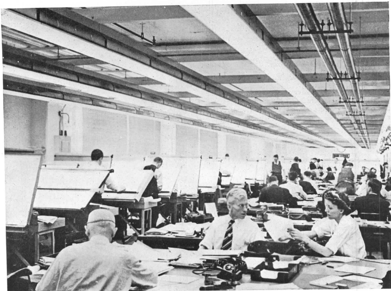
In this continuous row installation, one 40-watt fluorescent lamp in each troffer section provides an illumination of 50 foot-candles for this combined drafting room and office of a defense plant
