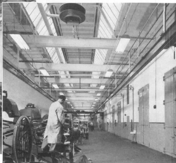
Architect and Engineer: Albert Kahn Associated Architects and Engineers, Inc., Detroit. General Contractor: Thorgersen & Ericksen Co., Chicago. Heating Contractor: S. J. Reynolds, Inc., Chicago. Photos by Hedrich-Blessing.
