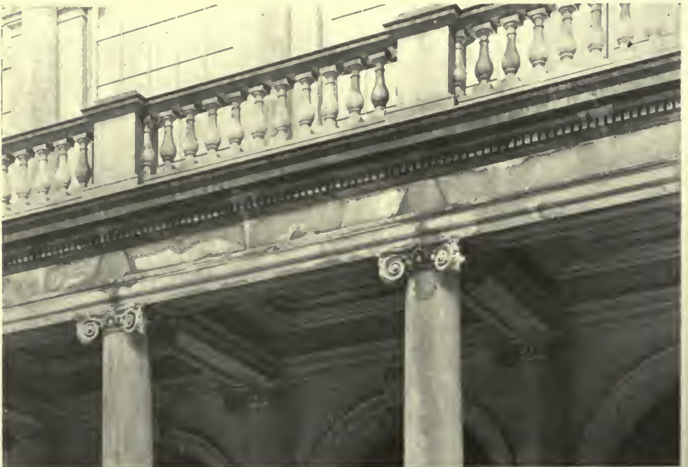
DETAIL AT PORTICO—NEW YORK CITY HALL. COMPARE THE DETAILS OF THE OUTER COLUMN CAPITALS WITH THOSE THAT HAVE BEEN PROTECTED BY THE ROOF.
