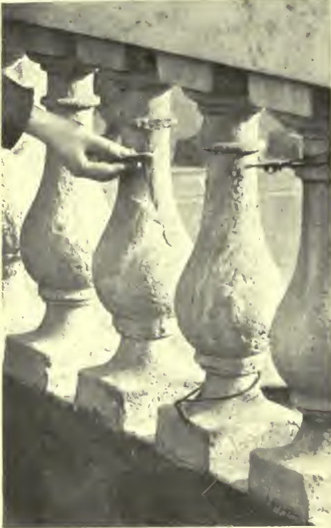
DETAIL OF BALUSTERS—NEW YORK CITY HALL. THE MEREST PRESSURE WOULD BREAK OFF ANY OF THE NECK MOULDINGS AS IT HAS DONE IN THE CASE SHOWN.
