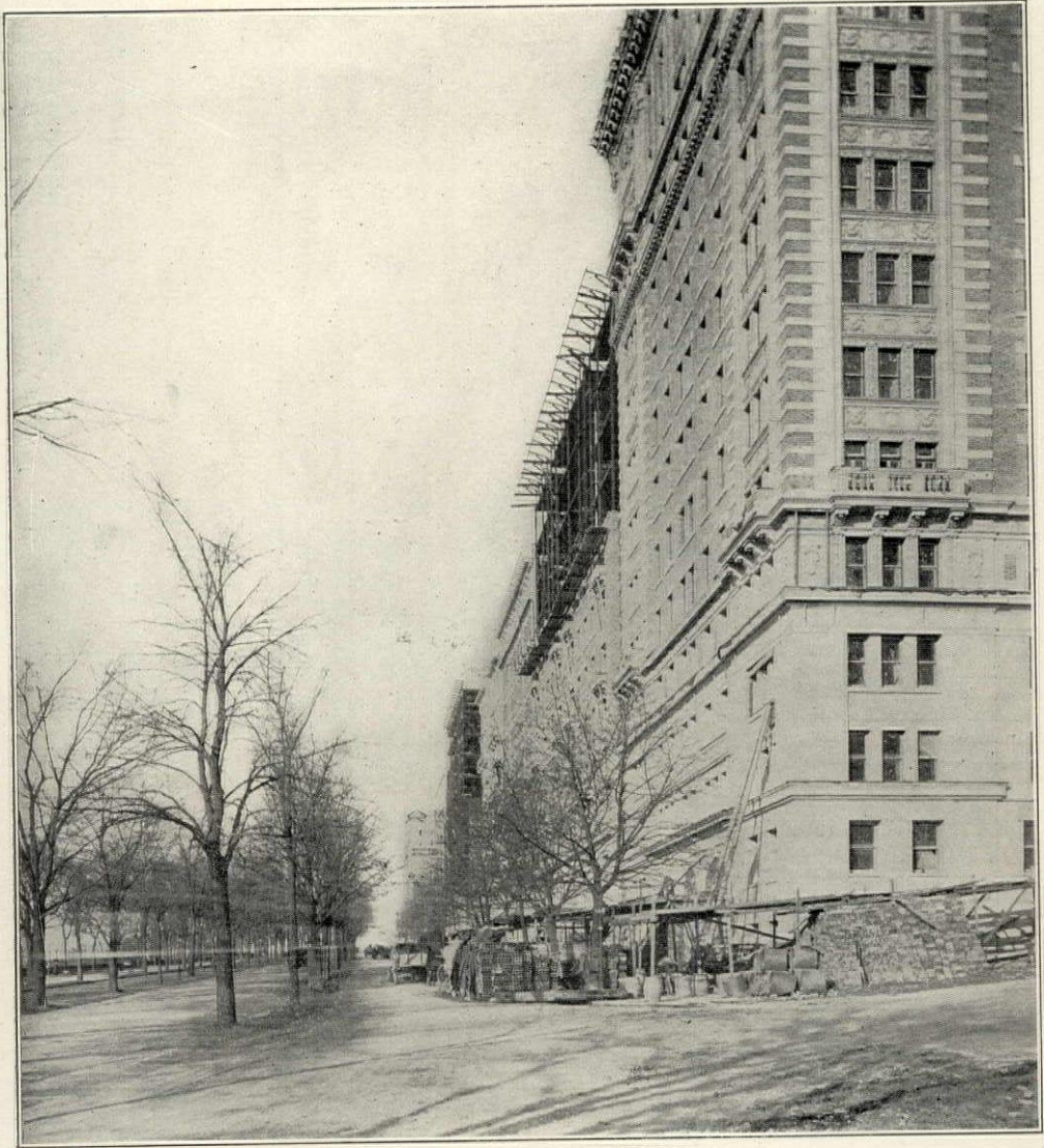
LOOKING NORTH ON RIVERSIDE DRIVE FROM 116TH STREET—ONE OF THE MOST ACTIVE SECTIONS IN THE FIREPROOF TYPE OF APARTMENTS.
